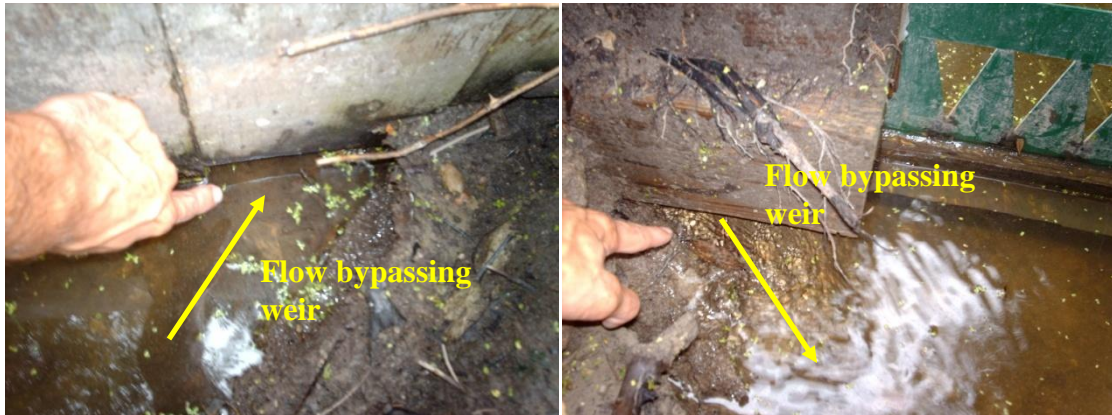
Figure 18. Scour hole resulting in water bypass of outflow weir.
