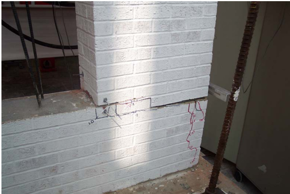
Figure 11: Rocking Mechanism and Limited Crack Width at 1.75 Drift Ratio
