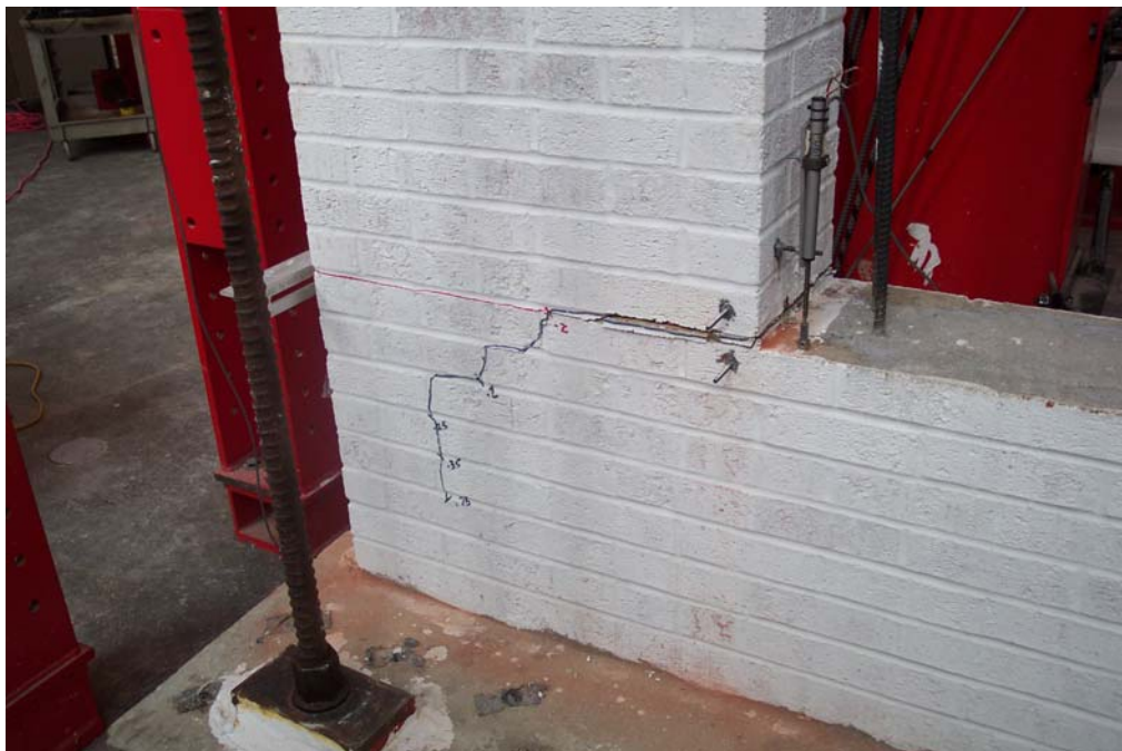
Figure 10: Reduced Crack Width at 0.75 Drift Ratio
