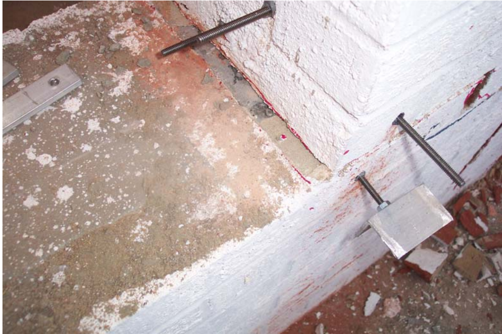
Figure 9: Observed Sliding of Masonry Wall at 1.75 Drift Ratio
