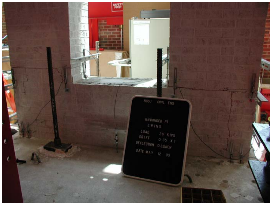
Figure 2: Formation of Base Crack and Vertical Crack at 0.35 Drift Ratio
