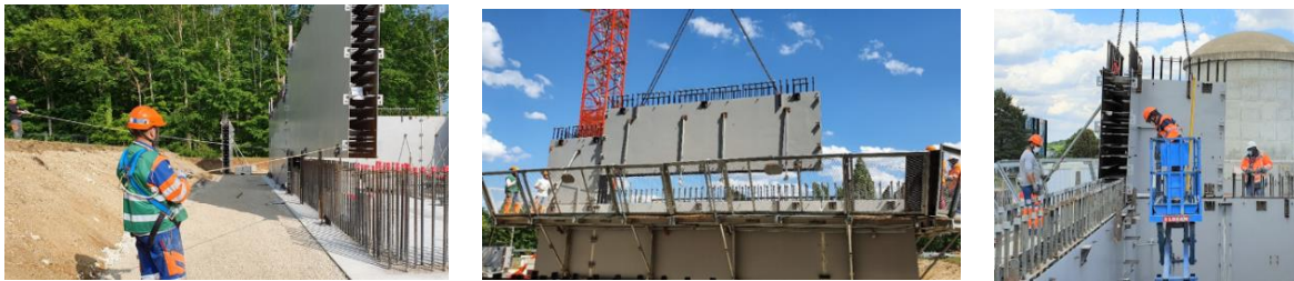
Figure 6. Wall module installation (level 1 on the left – level 2 on the middle and on the right)
