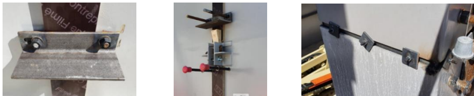
Figure 9. Joint sealing with timber formwork (left and middle) - with inner steel strip (right).
