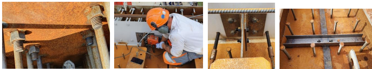
Figure 18. Slab T-stiffener connection to wall (left and middle) - Longitudinal joint sealing (right)
