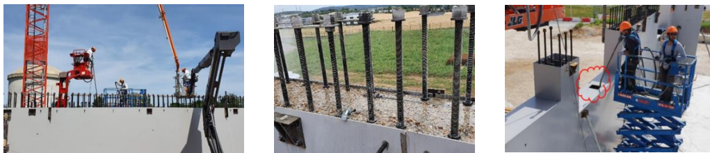
Figure 16. Wall concreting (left) - concrete top surface (middle) – vibration at large opening (right)
