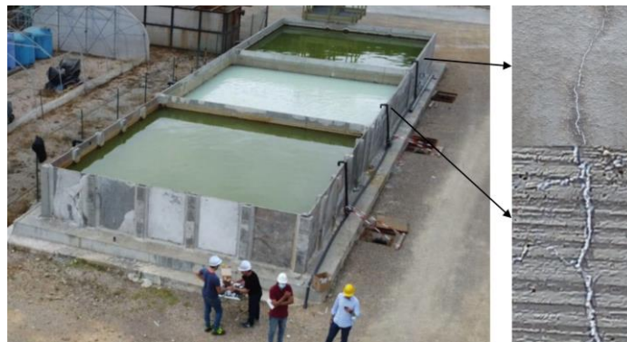
Figure 4. Filled water tanks and monitored cracks with sealing in a pilot testing.
