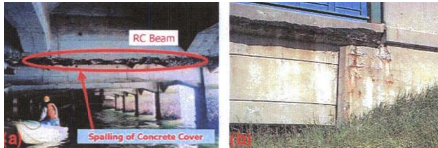
Figure 2. Corrosion of sea water structure (left) and bridge structure (right) (Naus, 2007).
