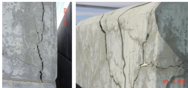
Figure 1. Concrete cracking at northwest (left) and northeast (right) corners (USNRC, 2024).
