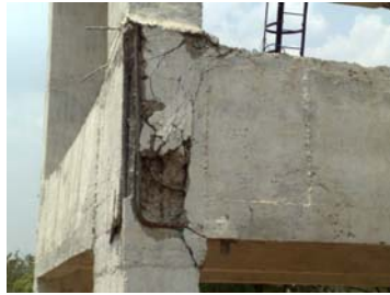
Fig.10 Joint failure of CL 19 at 1 st floor
