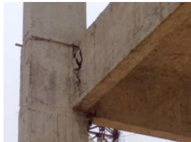
(b) Beam BF 223 at 1 st floor, torsion failure
