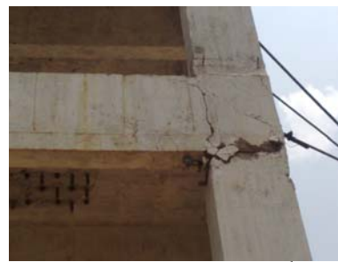
Fig.13 Joint Failure CL20, 2 nd floor
