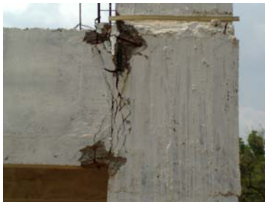
(a) Beam BF 205 at 1 st floor, flexure failure
