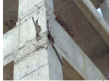
Fig.11 Joint failure of CL 19 at 2 nd floor
