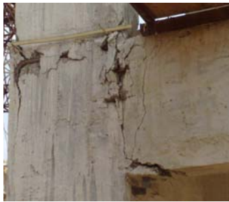
Fig.12 Joint failure CL16, 1 st Floor
