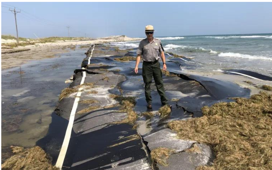
Figure 1.1: Superintendent David Hallac standing on a damaged stretch of State Highway 12 on Ocracoke Island (Credit: NPS)
