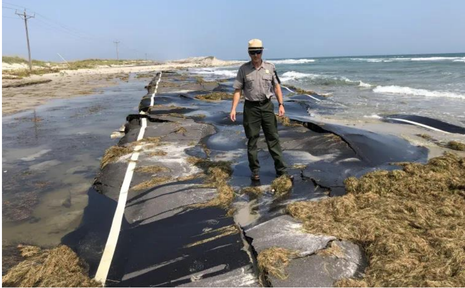
Figure 3.4: Superintendent David Hallac standing on a damaged stretch of State Highway 12 on Ocracoke Island (Credit: NPS)
