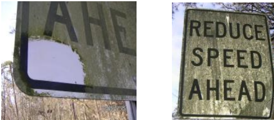
Figure 7.13. Dirt on Sign from Feed Mill (Before and After Cleaning)
