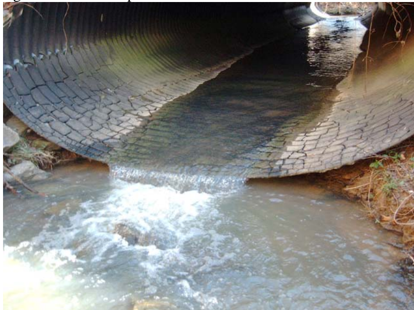
Figure 5. Perched Pipe Culvert.
