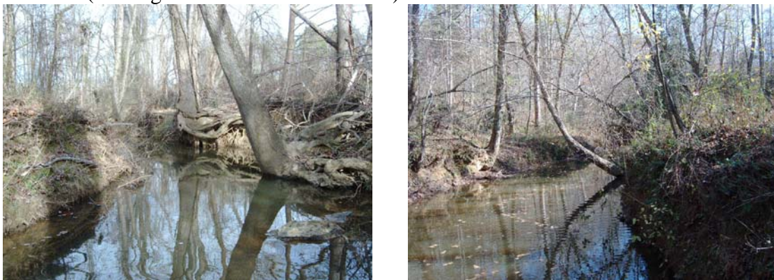
Figure 2. Photographs of Channel Widening, Incision, and Overhanging Trees (looking downstream from culvert).
