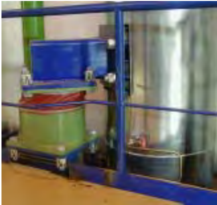
Fig. 1 VD-Damper Installed on Pipeline of NPP (Turbine Hall)
